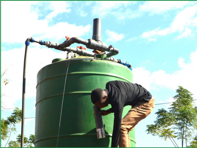
A snapshot of how the In-line chlorination device is installed
