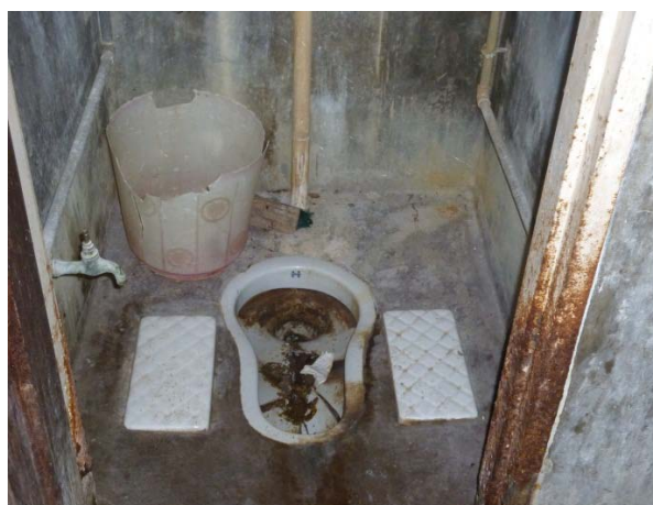
Images 1 and 2: Dirty toilet, no water, no door
